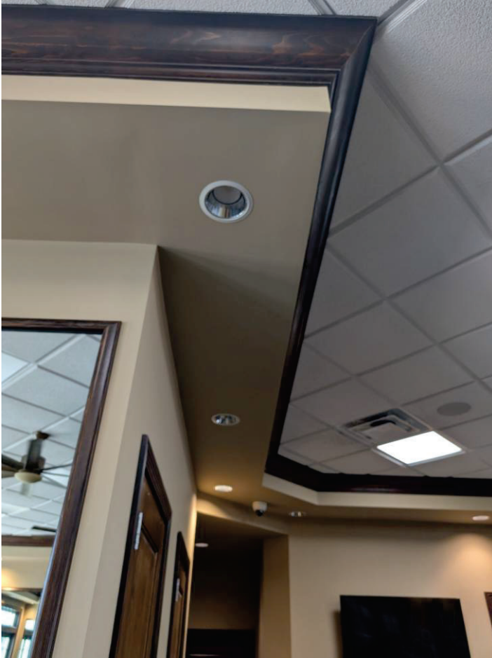
Figure 1. Existing Fitness Center recessed lighting.
