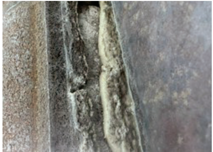
Oakmont - Underside of Coping Showing Gap
